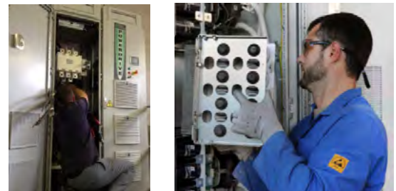
Diagnostics, inspections, replacement of power elements, substitution by new complete products
