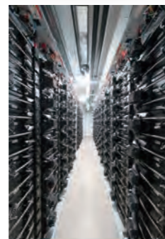
BESS (Battery Energy Storage System)
