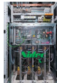
Power conversion system essential for the BESS
