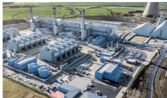
EDF Energy Renewables's West Burton Facility in Nottinghamshire, the UK, where Nidec ASI's BESS will be delivered for National Grid.
