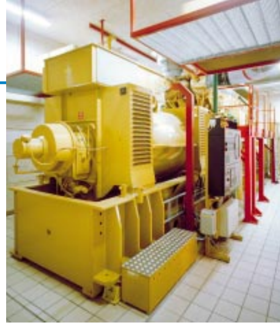
Denmark - Installation at Hvide Sande in 1994-95. Manufacturer of the power generating unit: Enmaco Motorer A/S - CATERPILLAR dealer. Gas engine type CAT G3616 SITA. Alternator LSA 56 UL 95 / 6 poles / 3845 kW / Medium voltage / Cos phi 0.9.
